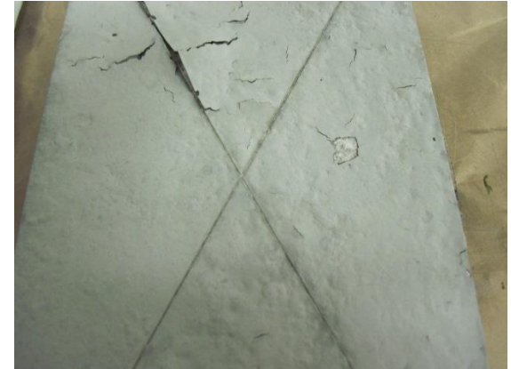
Poor NC Coating <1 Year; 2024 Al
